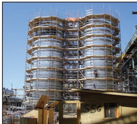
A tower built by Steeplejack at the Long Lake site near Ft. McMurray, Alberta, Canada, using Layher scaffolding.
